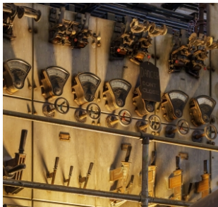
Powerhouse Switchroom Accepted Lyn Wilson
